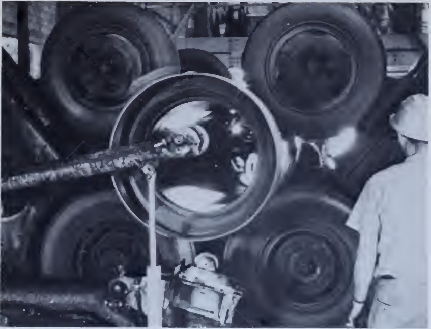
Figure 164. —A centrifugal method of manufacturing concrete pipe which also employs both direct compaction of concrete with a steel roller and mechanical vibration. P830-D-17221.
